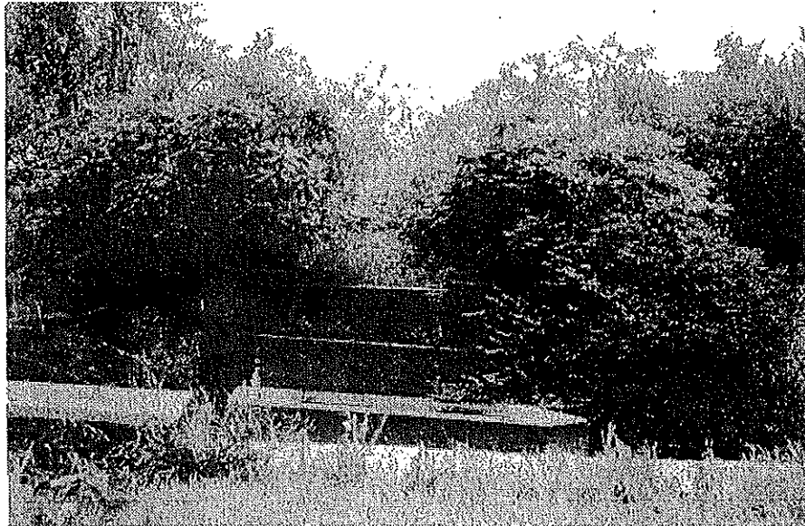
Concrete abutments are all that remain of a bridge that carried trains of the Erie Lackawanna Railroad across the Paulins Kill in Augusta.
